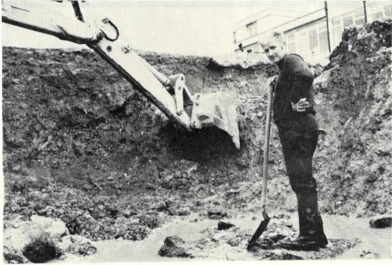
From a hole in the ground on the left, to a job well done a year later, below.
